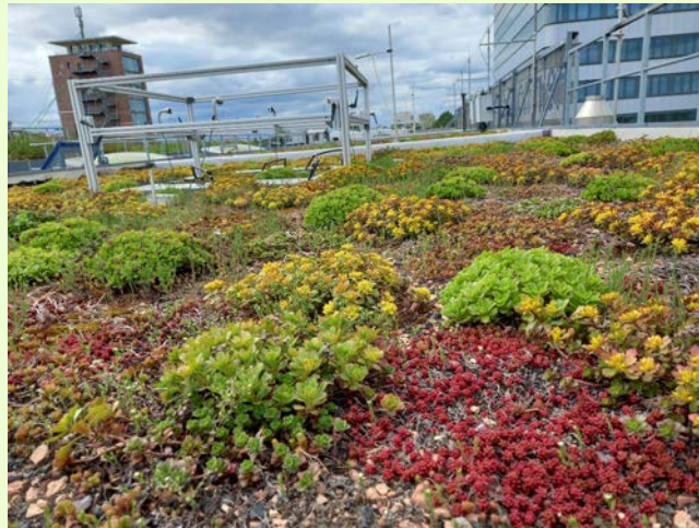
Extensive green roof in May 2024 (Photo: Lucie Moeller)
